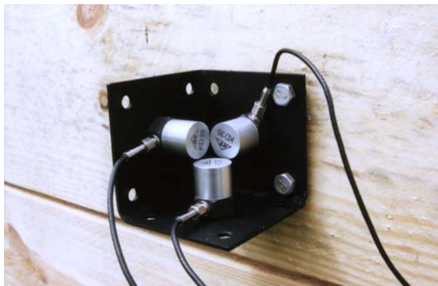
Fig. 23. Accelerometers installed on the bin wall
